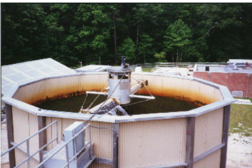
Typical motor-driven rotary distributor.
