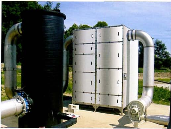
Photo-Catalytic Oxidation for exhaust deodorization
