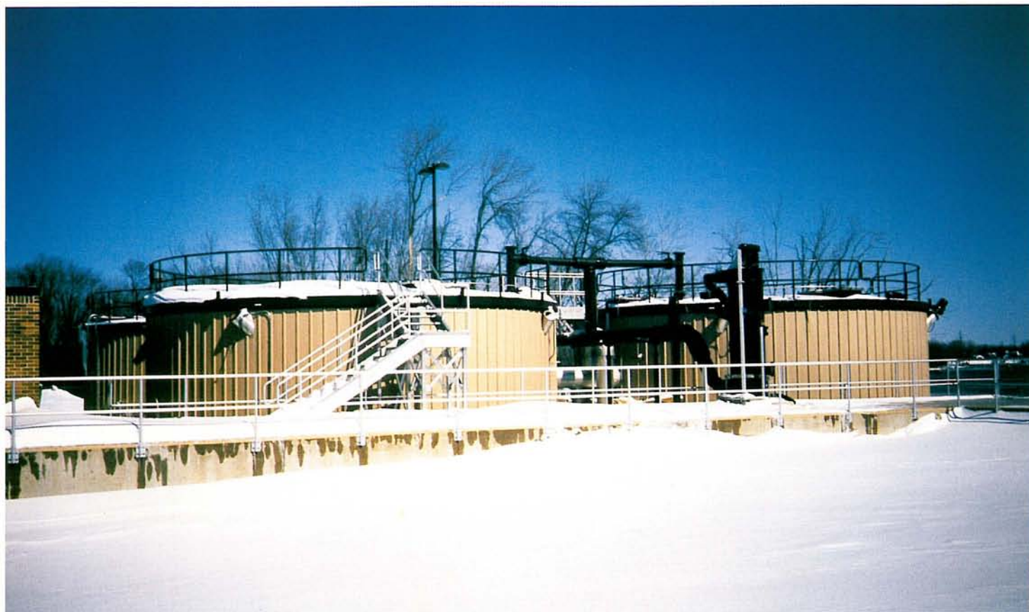
ATAD plant in Wisconsin, USA, for a total population of 48,000 (2.53 MGD)
